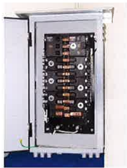
EG installed at building service entrance
