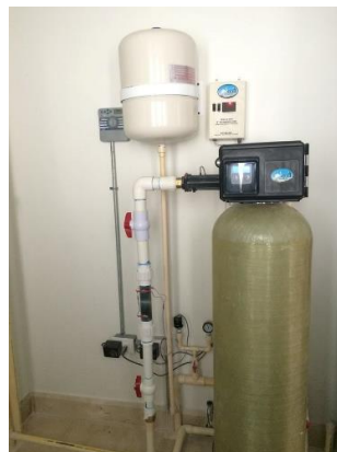
Light Commercial System Cistern and City Water Blend Yucatan, Mexico
