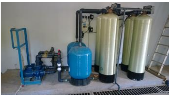
Quad Commercial System Serving Bottled Water Lagos, Nigeria 10,000-12,000 GPD
