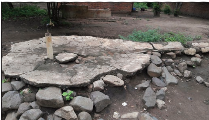
Broken down tap in Mbadzi Scheme (2015)
