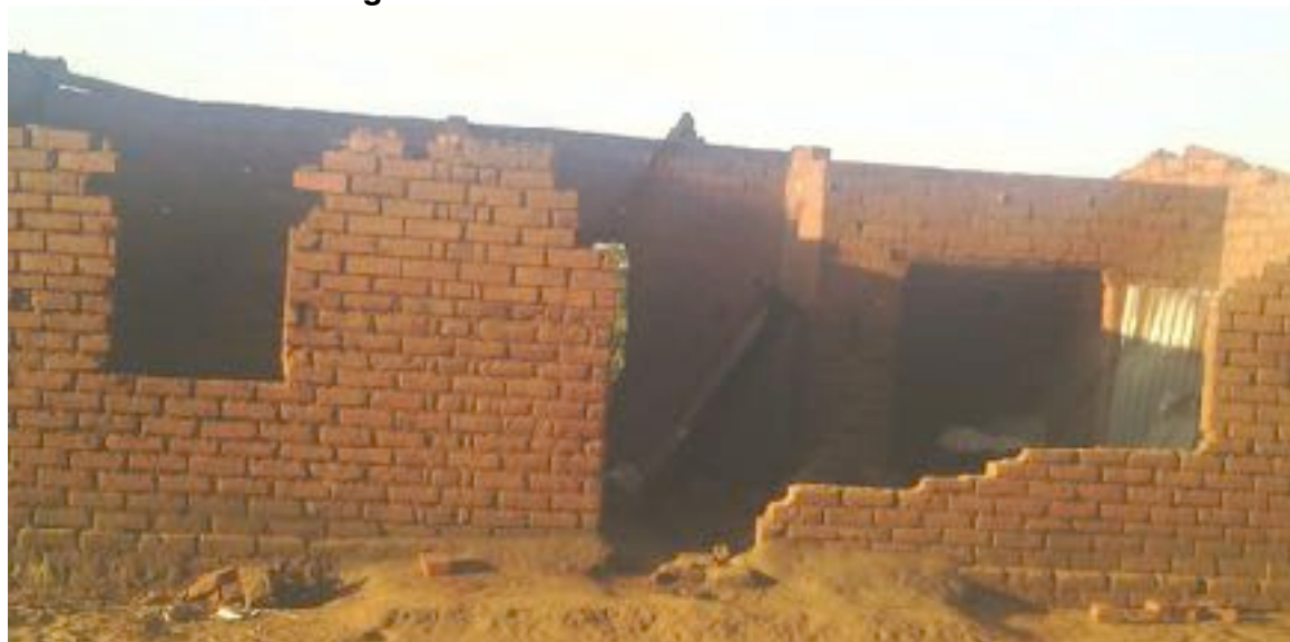
Photo 1: A storm damaged home
